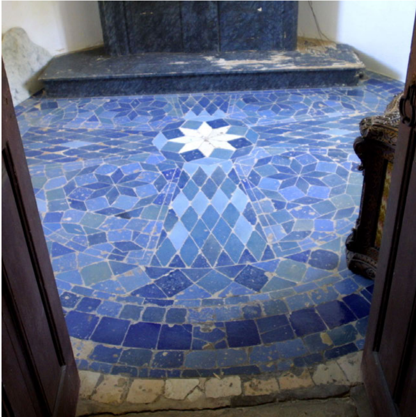
Figure 2. A view of the floor as it originally was, seen from the door, showing the narrow strip of rectangular tiles around the step to the altar (image © Associação de Colecções | The Berardo Collection).
